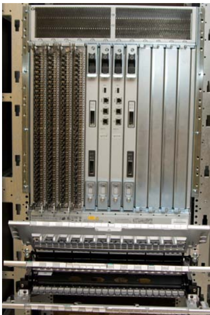
Figure 8. Installed patch panels (below cable comb)
