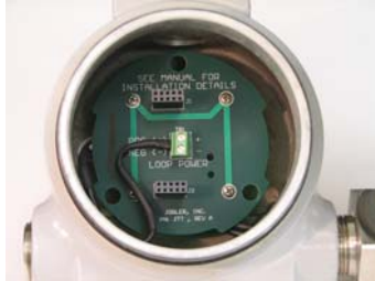
Photograph No. 2 Termination Board
