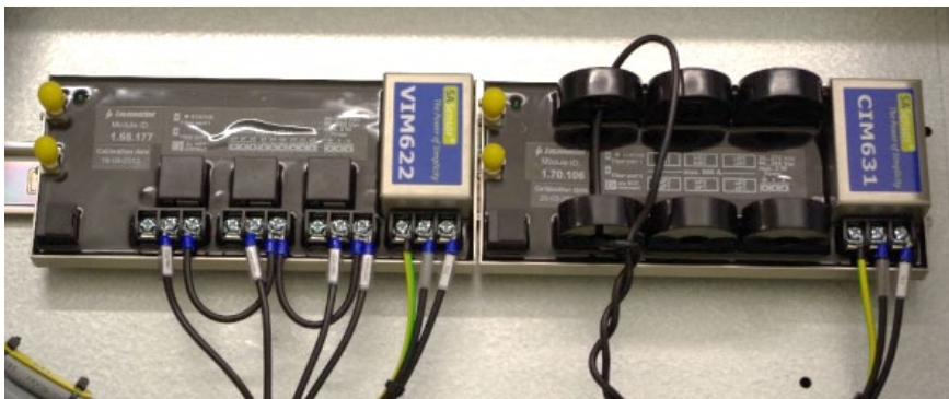
SASensor modules installed in one of the primary switchboard bays
