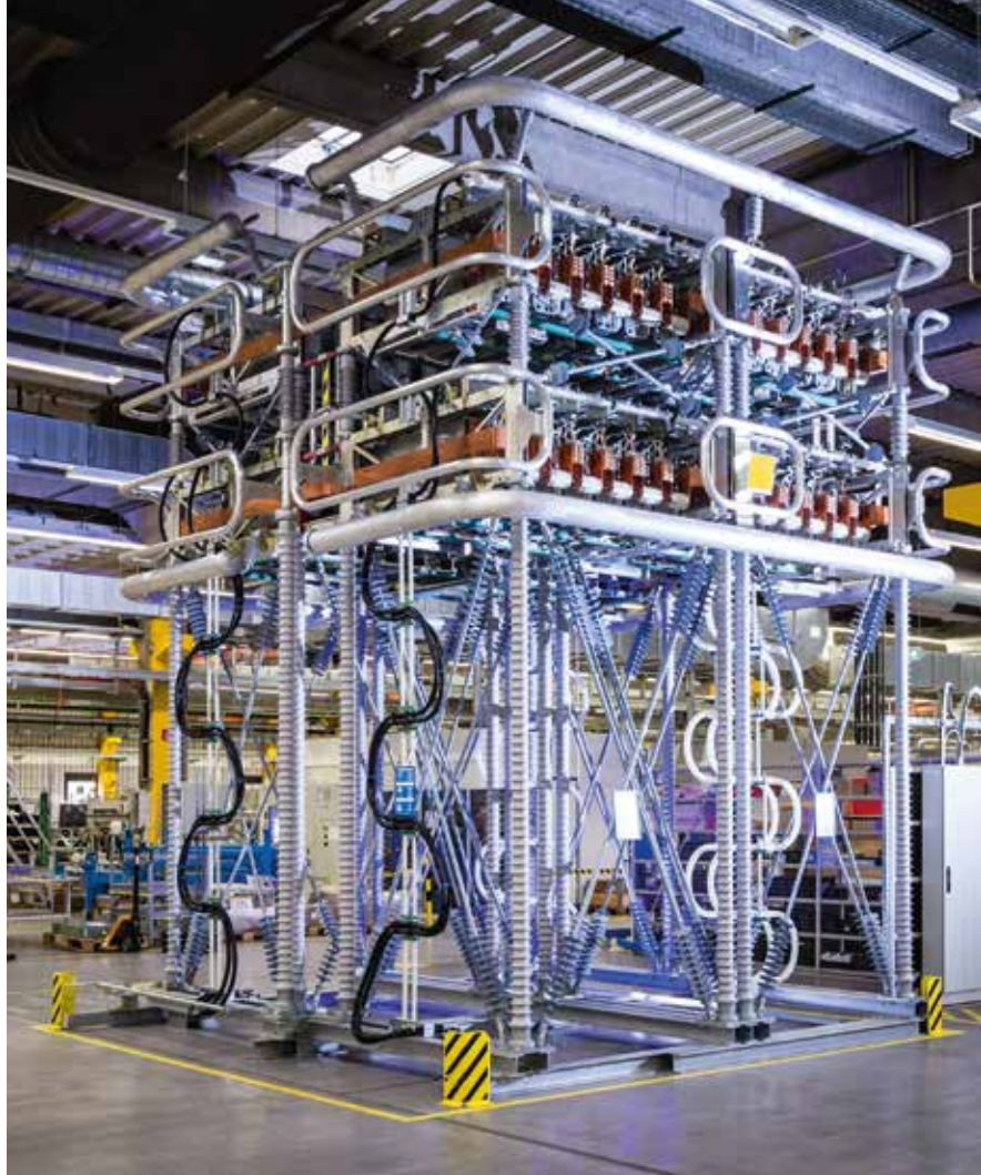
Converters in onshore stations turn direct current coming in from sea or land into alternating current.
