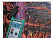
Fiber optic power test
