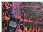
Fiber optic power test
