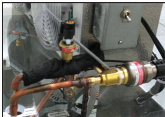
Figure 3. Evaporator line with insulating tape over sensor.
